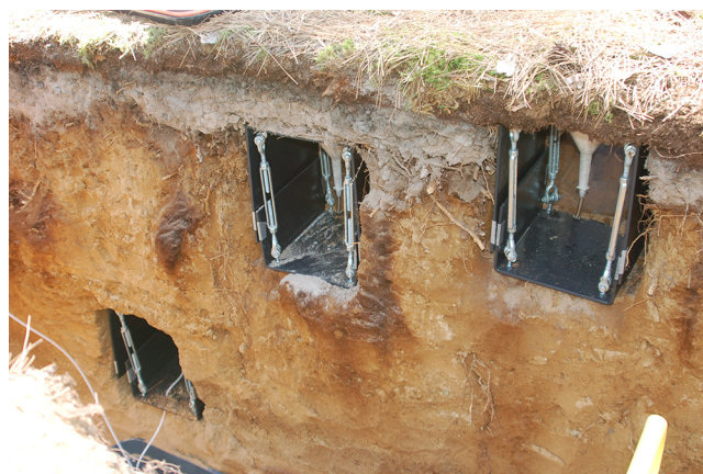
Fig. 1. Photograph showing the location and installation of zero-tension lysimeters below the Oe horizon (right), E horizon (middle) and lower B horizon (left).
